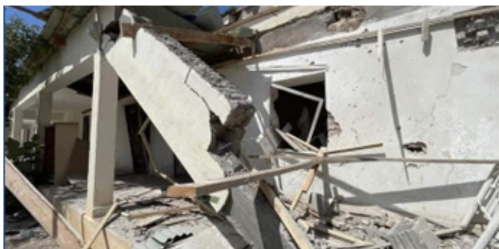
Health facility destroyed in Laascaanood
